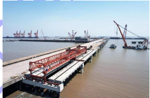
图 9 浮吊配合架桥机箱梁安装 Fig. 9 Coordinated erection of box girders using floating crane and bridge erection machine
