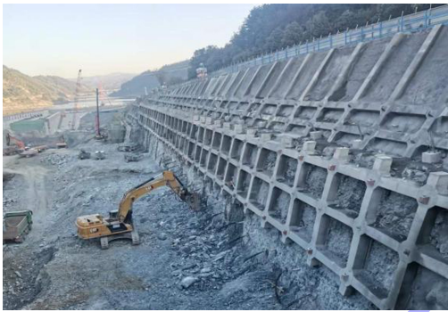
图5 “框格梁+预应力锚索”支护效果 Fig.5 Supporting effect of “frame beam+prestressed anchor cable”
